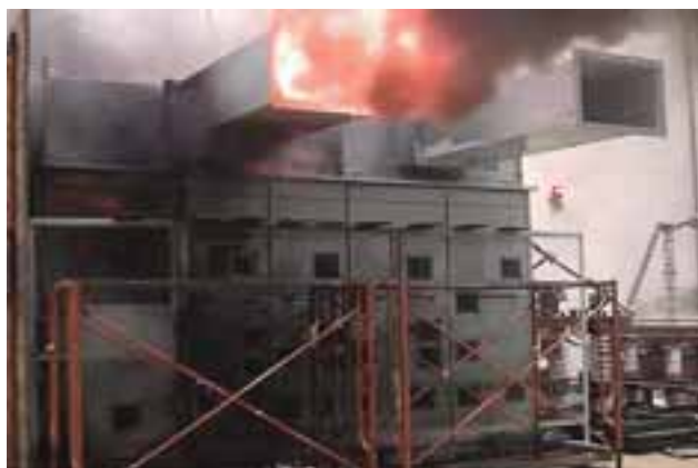
Arcing due to internal fault test
