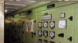
Generator Control and Power Management System
