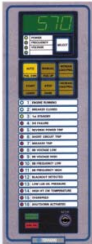
Operator Panel for one Generator Set
