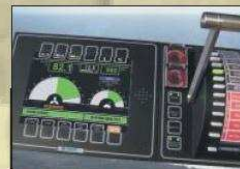
Propulsion Control System
